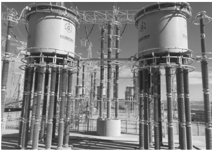
图8 \pm 800\text{ kV} 灵州换流站 750 kV TRV 电容器现场运行照片 Fig. 8 Site operation picture of 750 kV TRV capacitor at \pm 800\text{ kV} Lingzhou converter station
